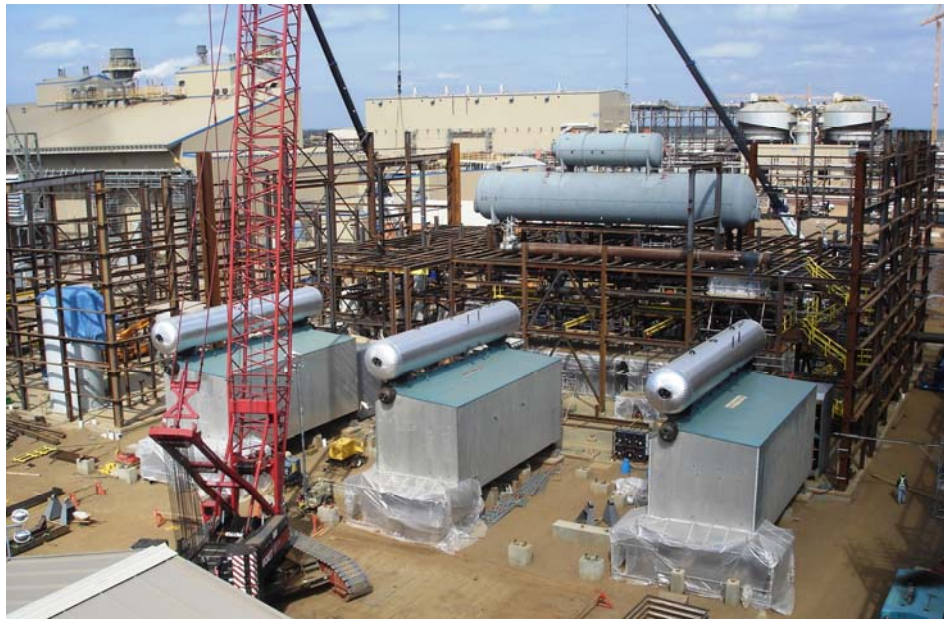
Fig 4: (Addendum) Elevated Drum package boilers, each rated for 426,000 lb/hr, shown during installation. A total of five(5) units were supplied on this project for a major oil producer.
